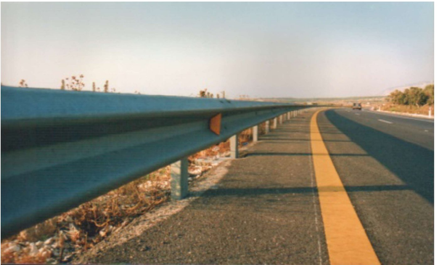
Road final shape - Steel guard rail - Wearing course - Edge marking yellow line
